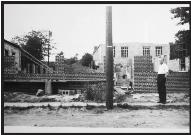
Stephan J. Schaffan Sr. oversees the construction of the first Atlas track factory in Hillside NJ.
